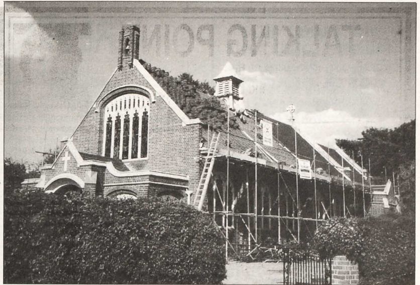
Our picture shows work in progress on the nave roof at St Barnabas Church during August J. Hardy
