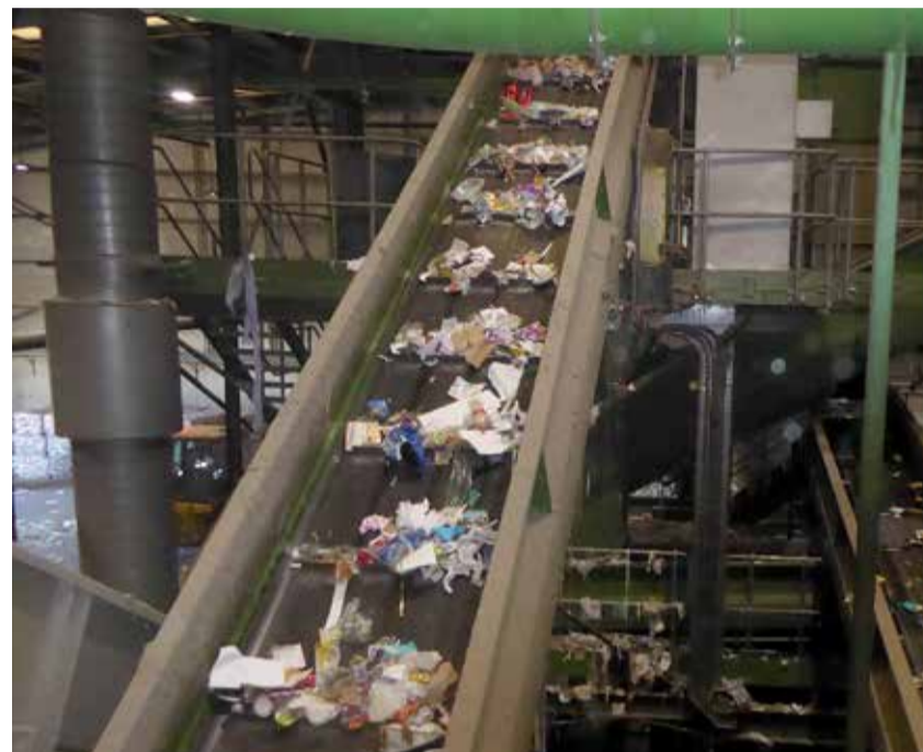
Conveyors of good waste
